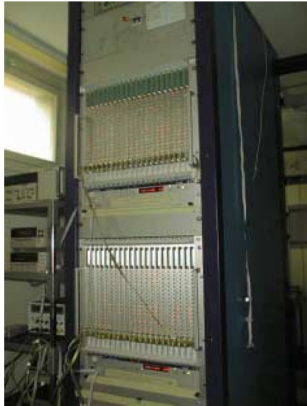
Figure 2- Front view of rack fully equipped with 9U load cards.
